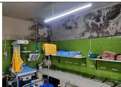
Figure 5.6: Dampness in walls in the Labour room at THQH Vythiri (29 November 2022)
