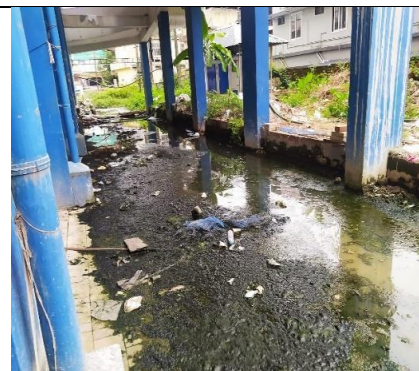
Figure 5.5: Clogging of waste water in DH Tirur (25 November 2021)
