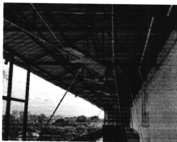
Picture 4.2: Remnants of false ceiling hanging from the roof at Pareeksha Bhavan. 16 October 2018
