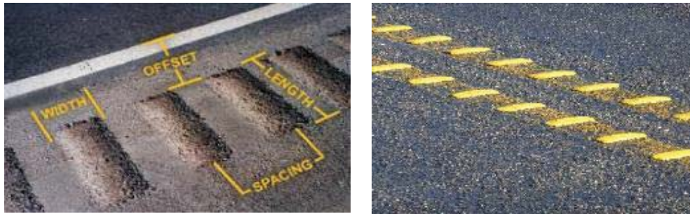
Rumble strips (a) bitumen & (b) yellow line at inside side edge of paved shoulder
